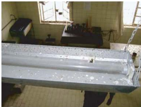
Non-functioning, not cleaned UVGI fixture
