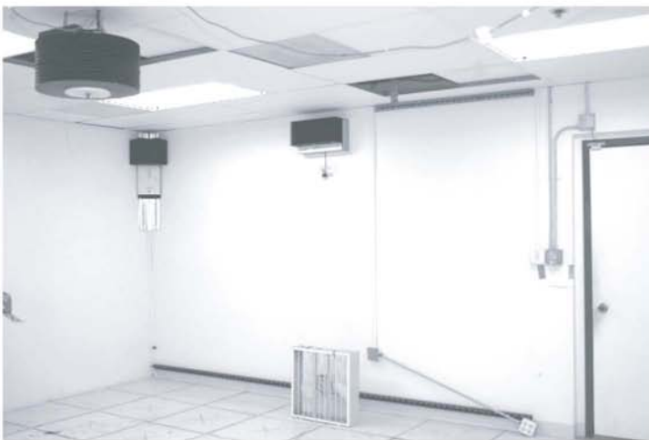
Corner wall and ceiling mounted UVGI fixtures
